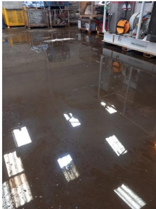
Photo 30. Sheen visible in standing water in Building 54.
