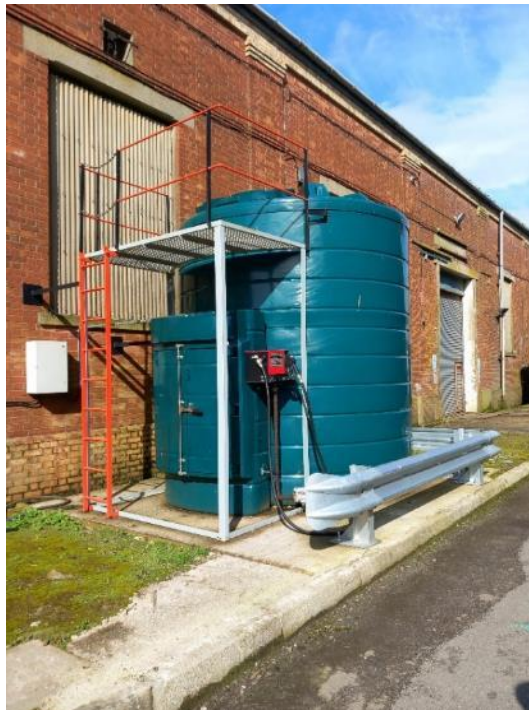
Photo 18. Kerosene tank located to the west of Building 428.
